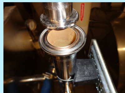
Rouging in a stainless steel pipe of an ultrapure water pipe
